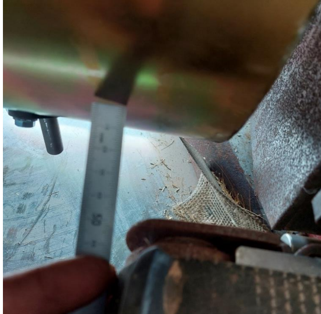
Figure 9: Excessive feed drum clearance to side drapers
